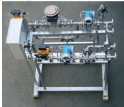
Regulation unit with wiring to terminal boxes
