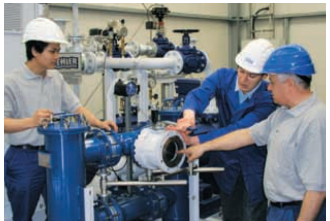
Commissioning and training by Lechler staff
