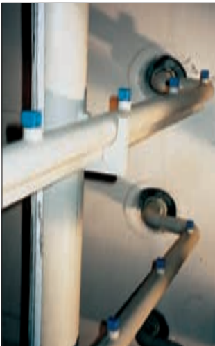
Detail nozzle spray system
