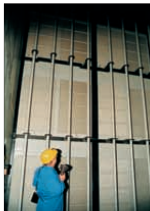
Installed LTH 100 in a flue-gas desulphurization plant
