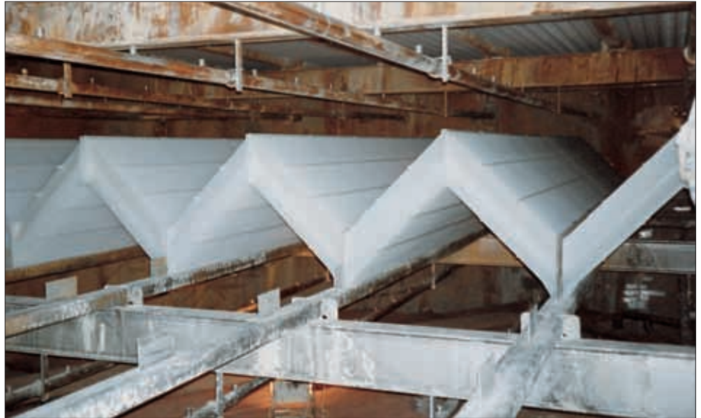
LTV 110.33.-B in a wash tower
